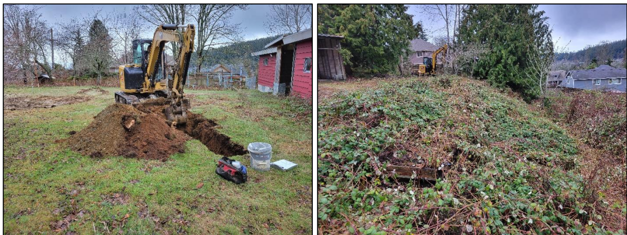
Image 1 (left) and Image 2 (right) – General surface conditions of the subject property. Image 1 is TP-2 in-progress facing southwest. Image 2 showing the slope area at the northern edge. Perspective is from the northeast corner facing southwest. Photos taken January 27 th , 2023.
